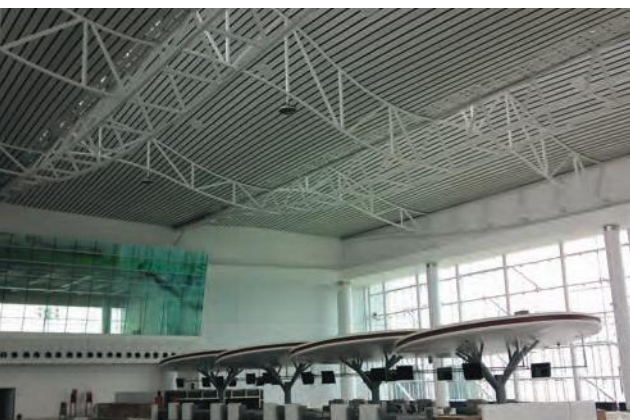
Sepinggan Airport Balikpapan, Indonesia 150C Ceiling
