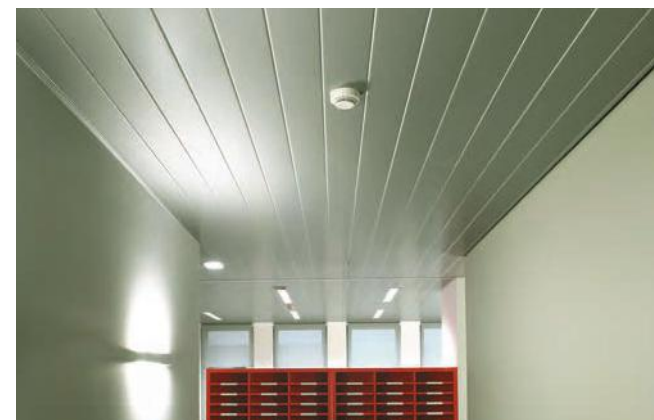
InBev Brewery, Belgium 150C ceiling
